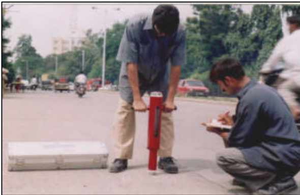
↑ M Type Rebound Hammer Test used for assessment of in-situ strength of rigid pavement.
