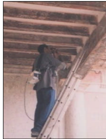
↑ Endoscopic inspection to check the condition of incased wooden joists mainly in heritage structures.
